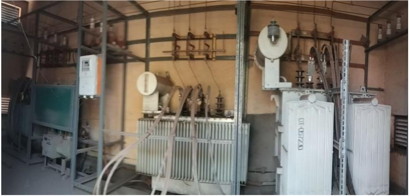
Figure 3:2 Assela Malt Factory power house
