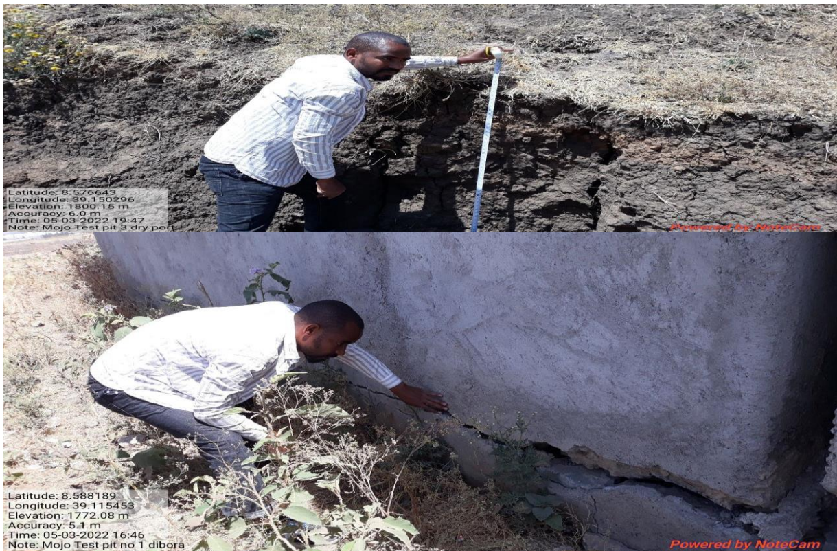
Figure 12: (a) Typical Test pit Depth b) Typical crack of Building due to Expansive soil around study area
