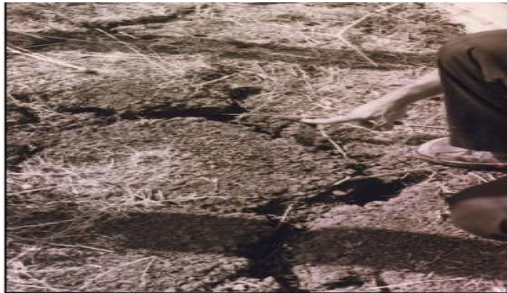
Figure 5: This crack is at least 32 inches deep. The yardstick was easily inserted to this depth; narrower, less straight cracks may extend much deeper (J. David Rogers, Robert Olshansky, et al).
