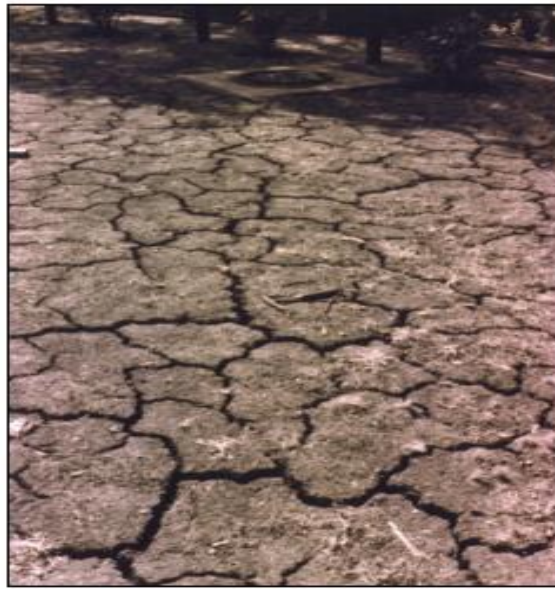
Figure 4: Polygonal pattern of surface cracks in the dry season. These cracks are approximately one inch wide at the top. Note sewer manhole in background (J. David Rogers, Robert Olshansky, et al).
