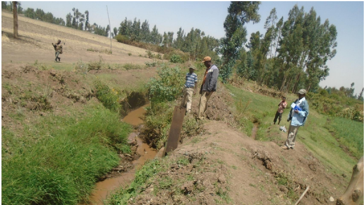
c. broken unlined canal at ketar i
