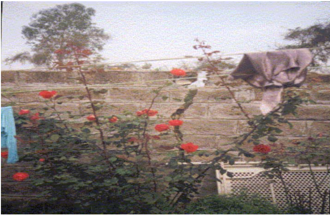
Figure 1.5. Tilting and sever crack of masonry store fence in the study site
