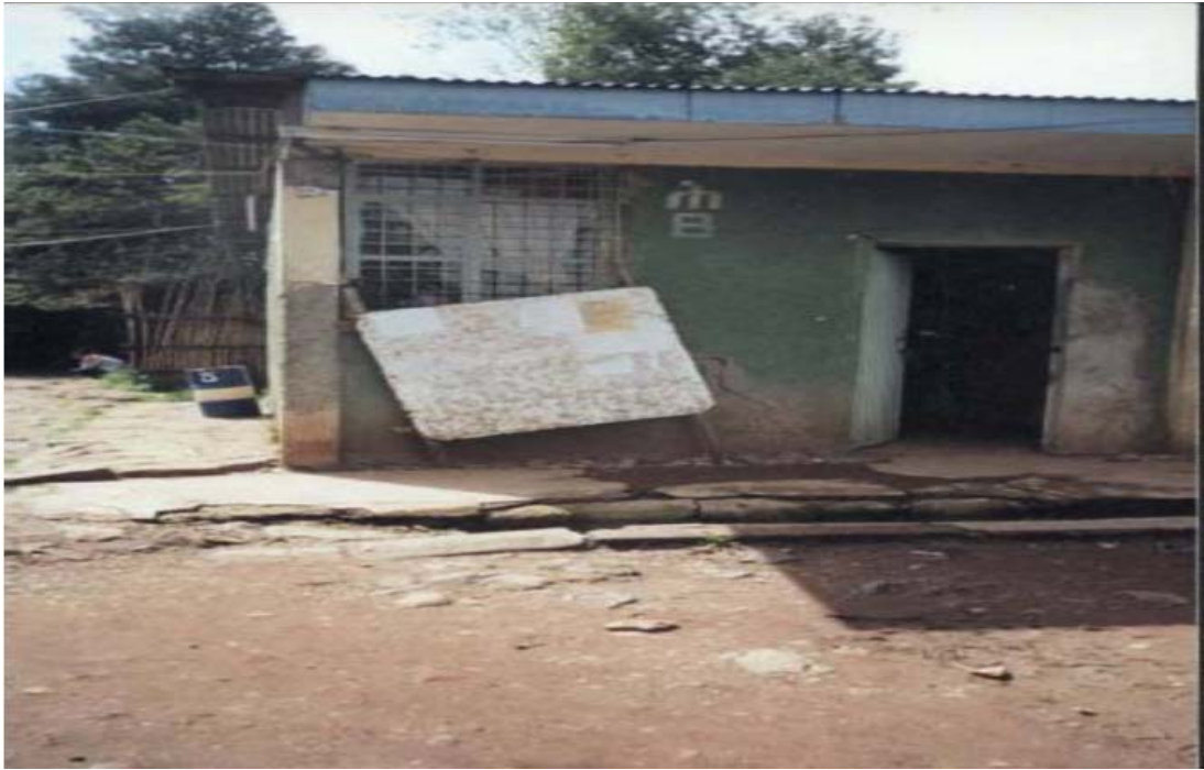
Figure 1.3. Detachment of tie beam and column in Gelan senior secondary school classrooms.
