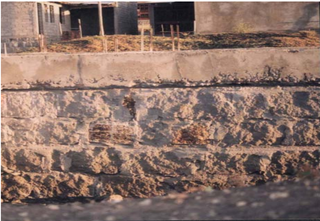
Figure 1.4. Settlement of masonry wall below grade beam in Gelan area around the municipality
