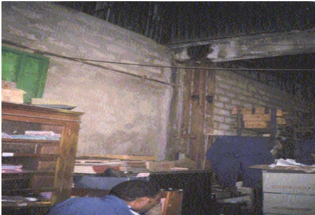
Figure 1.2. Shear of tie beam in Gelan city car parking basement building around the asphalt area
