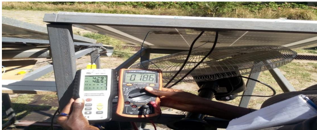
Figure: 4. 7 Voltage and temperature measurement of PV modules cooled by air.
