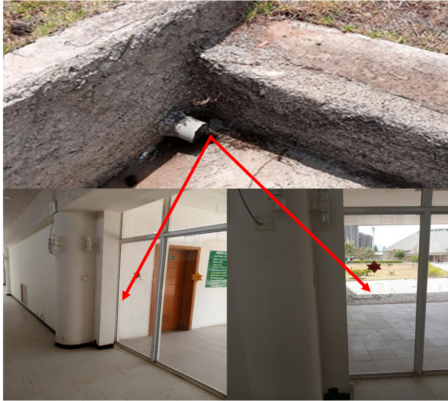
Figure 15: The drainage pipe from the green roof into drainage system
