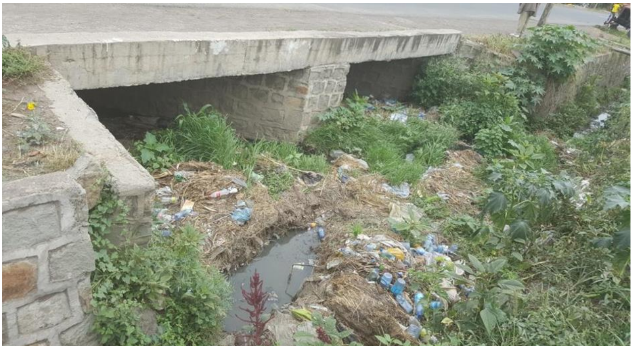
FIGURE 4 5: Culvert outlet with accumulated solid waste. (Source: field surveying).
