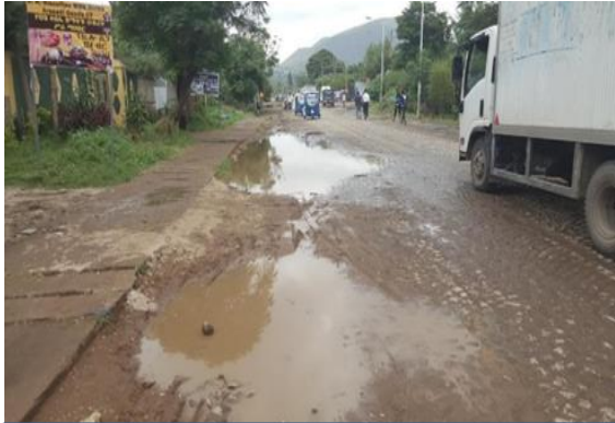
FIGURE 4. 15: Drainage & Slab Cover do not receive surface drain
