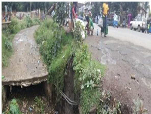
The drainage line in front of bust station seriously blocked with silt-up of mud and waste
