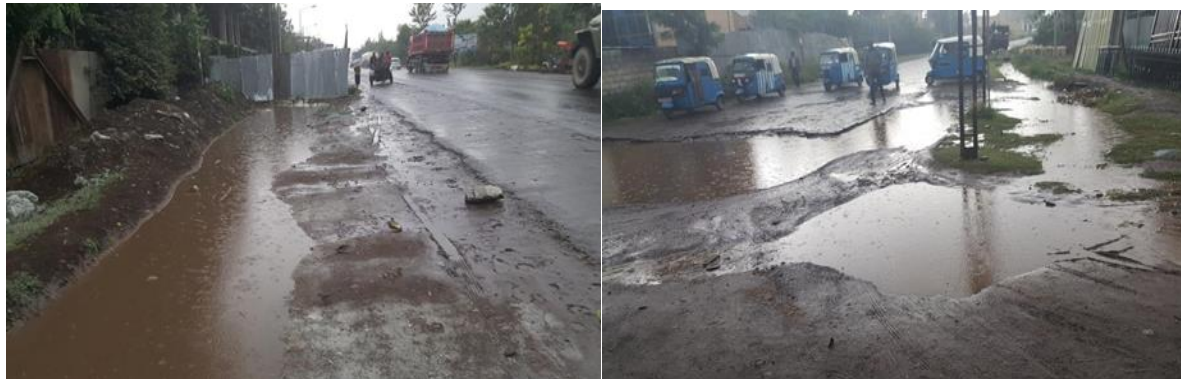
FIGURE 4 .6: No Surface and Side Drainage on main road around Lemlem area Source (Source : field surveying).
