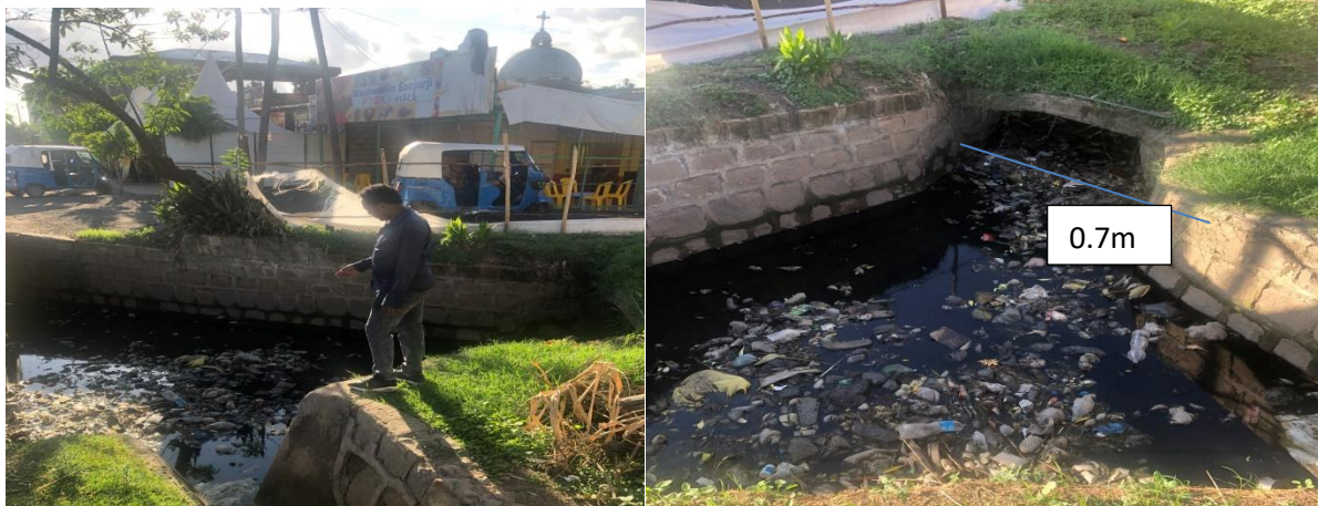
Figure 4.17 Garbage dumping in drainages canals and inadequate out let
