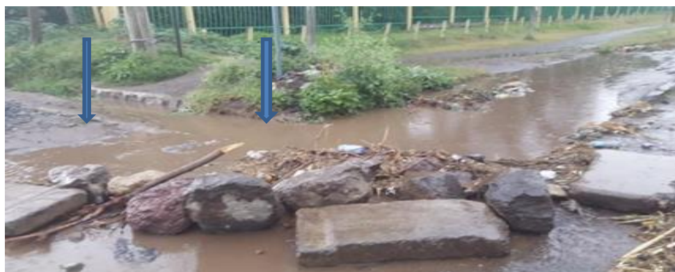
FIGURE 4 .9 challenge of existing drainage line. (Source: field surveying).
