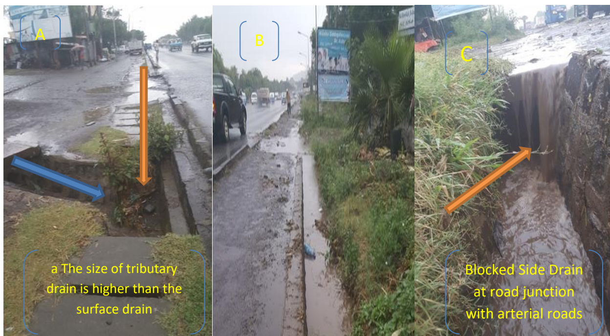
FIGURE 4 .8 challenge of existing drainage line (Source: field surveying).
