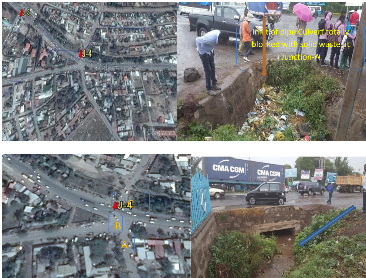
FIGURE 4.18 Inlet of pipe Culvert totally blocked with solid waste Junction-A. (Source: field surveying and from GIS).
