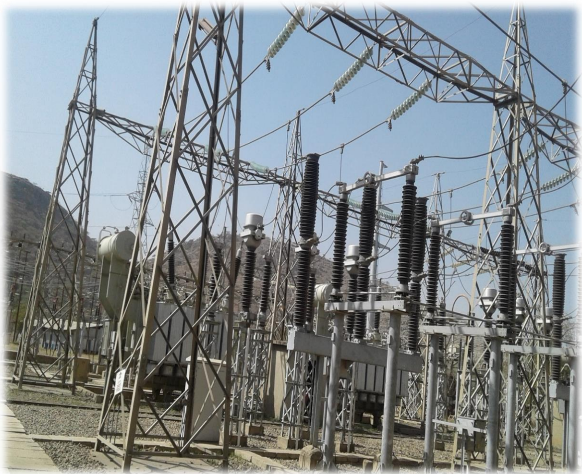
Figure 3.3: Dire Dewa Substation I [Source: Study Area]
