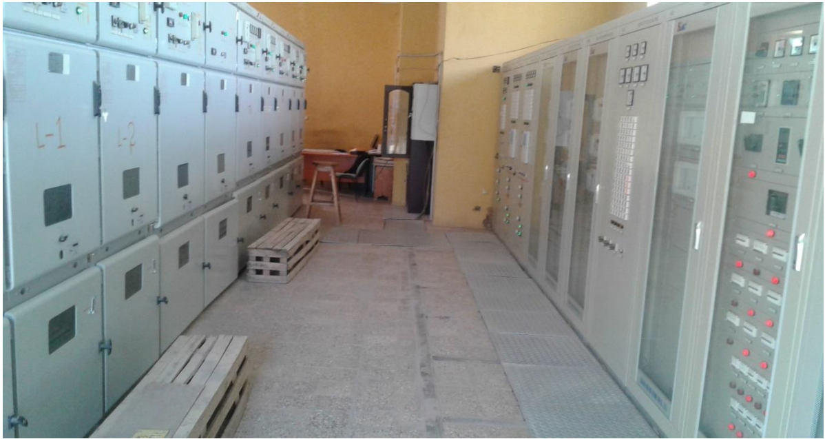
Figure 3.2 Partial View of DD Substation I Control Room [Source: Study Area]
