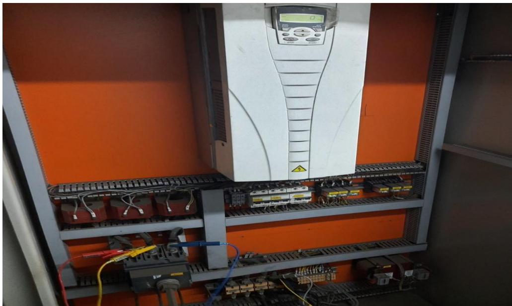
Figure A.6 Connection of Harmonics Analyzer on voltage supply side of VFD drive
