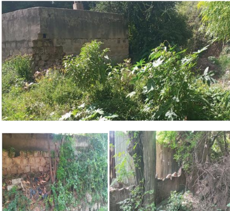
Figure 28 Impact on structure and residences 01 (Source: Author)
