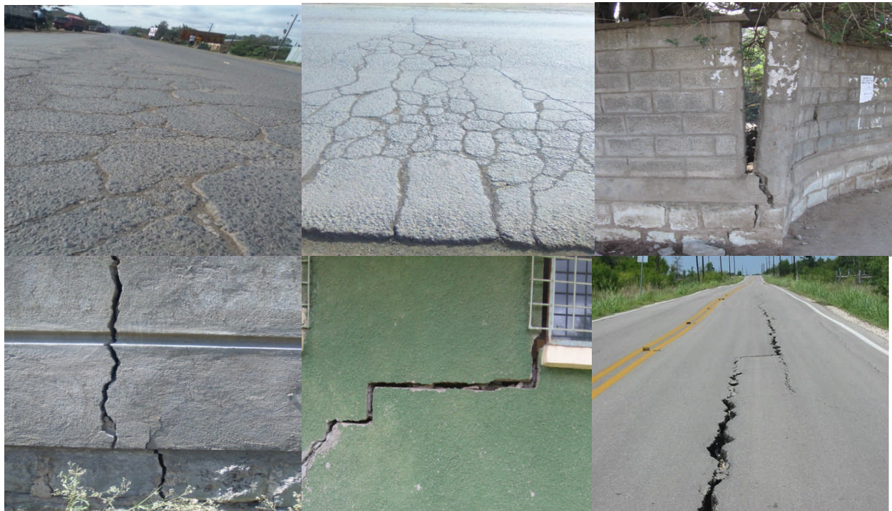
Figure1.4: Deformations and crack problems on study area section due to presence of expansive soils beneath subgrade and foundation soil respectively (Samson Y., 2017, Affework S., 2004).
