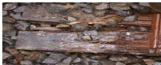
Figure 1.4. Rotting of the sleeper failing old railway found Adama
