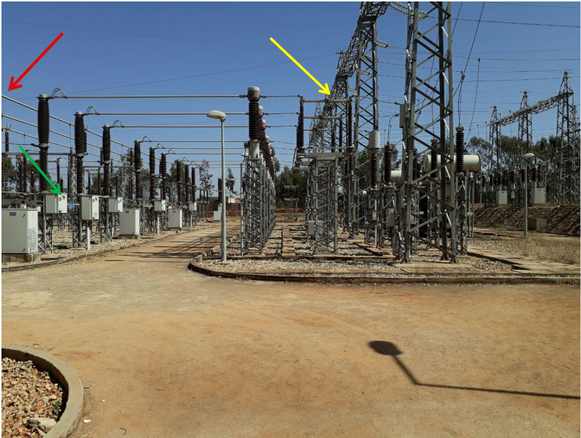
Figure 3.3: Harar Substation III [15]
