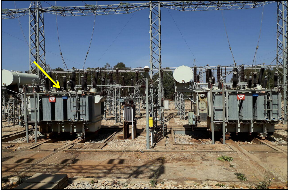
Figure 3. 4: Harar Substation III three winding Power transformer [15]
