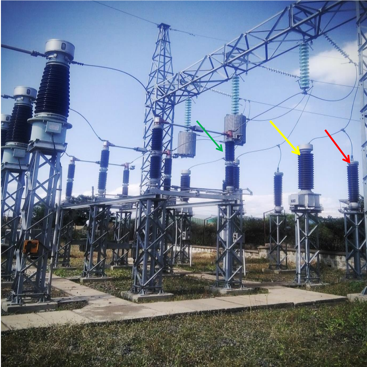
Figure 3.2: Harar Substation III incoming side [15]
