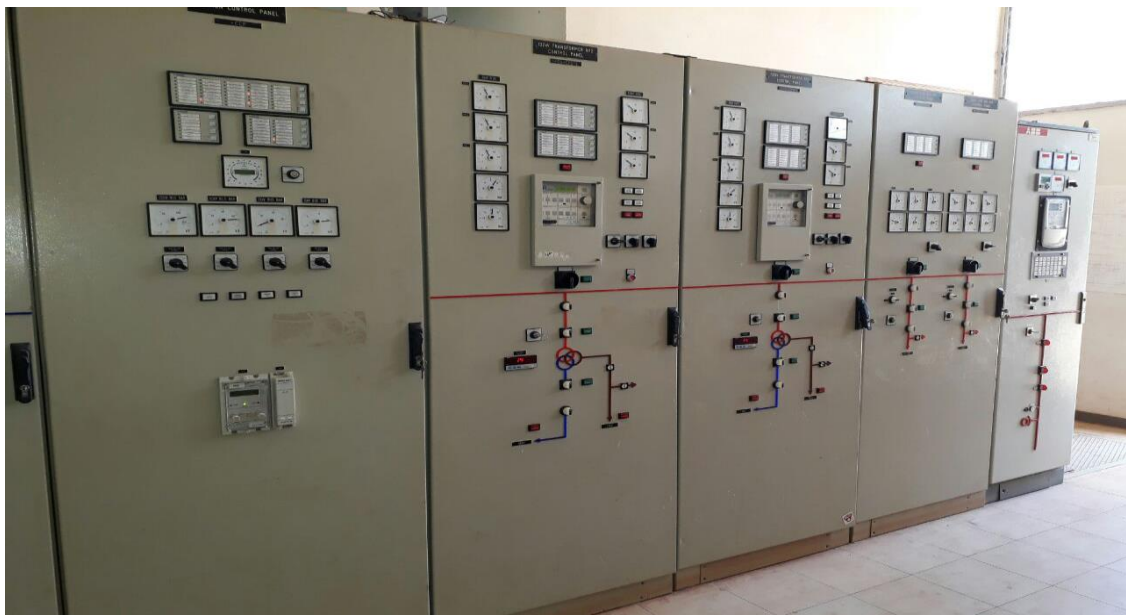
Figure 3.5: Partial view of Harar Substation III Control Room [15]
