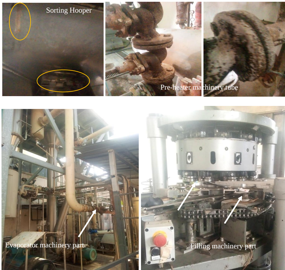
Figure 3.3 Corroded machinery parts in MFVPP
