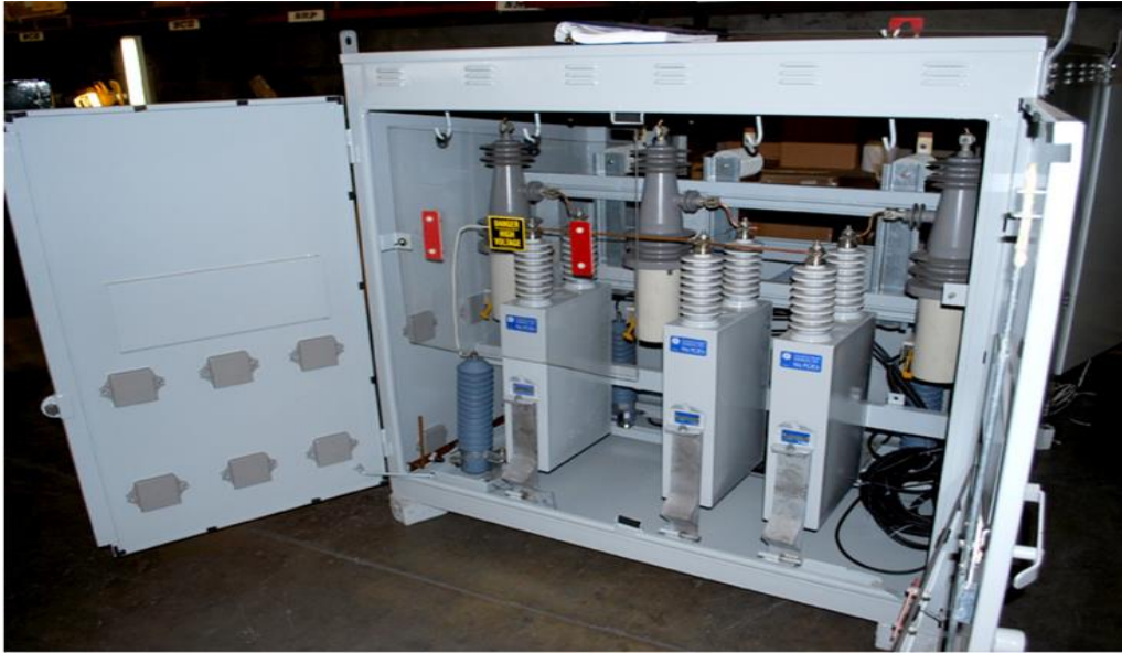
Fig 2.8: Custom pad mounted capacitor bank (photo credit: Scott Manufacturing and Engineering Power cap Capacitors Pvt. Ltd)
