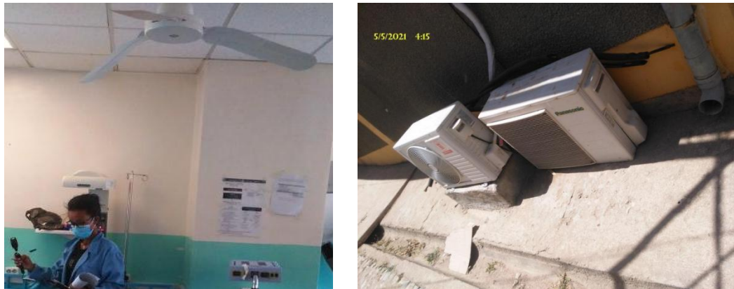
Figure 23 Existing cooling facility used.
