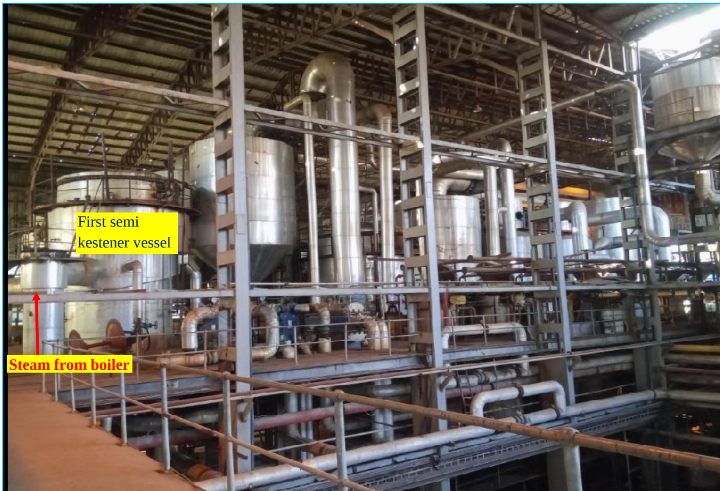
Appendix 4.6 Image of evaporation unit of wonji/shoa sugar factory
