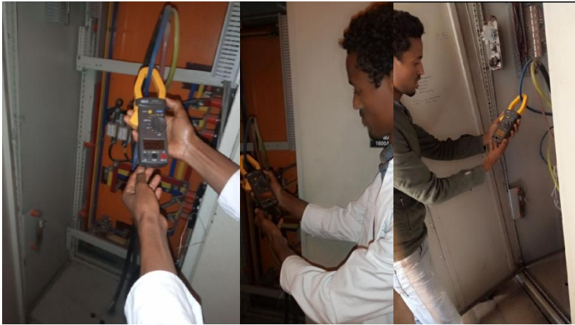
Figure 3.9: Measuring of current load by clamp meter for weighed raw juice pump motor
