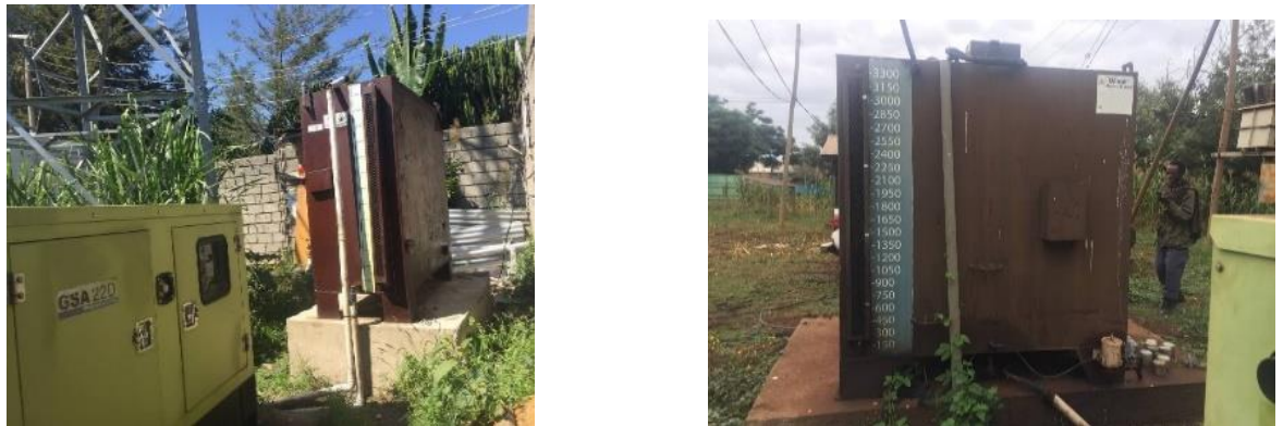
Figure 1. 1 Manual fuel level determining of BTS diesel generator fuel tank
