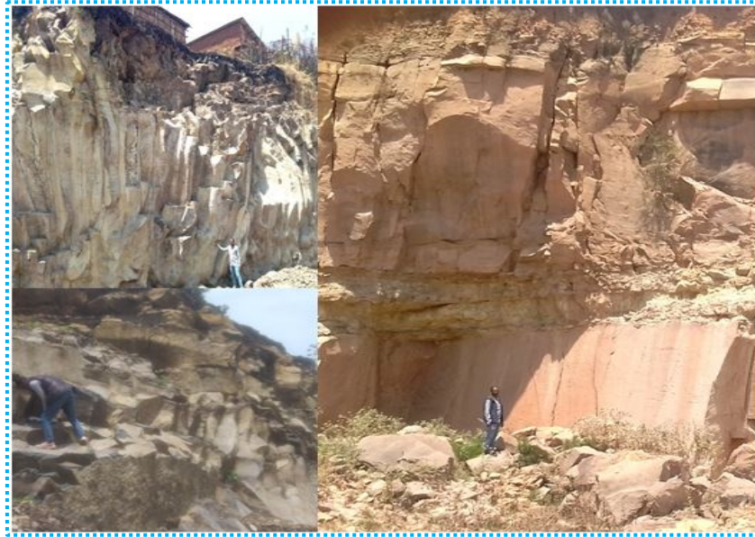
Figure 5.9 Rock slope falls sliding of the study area
