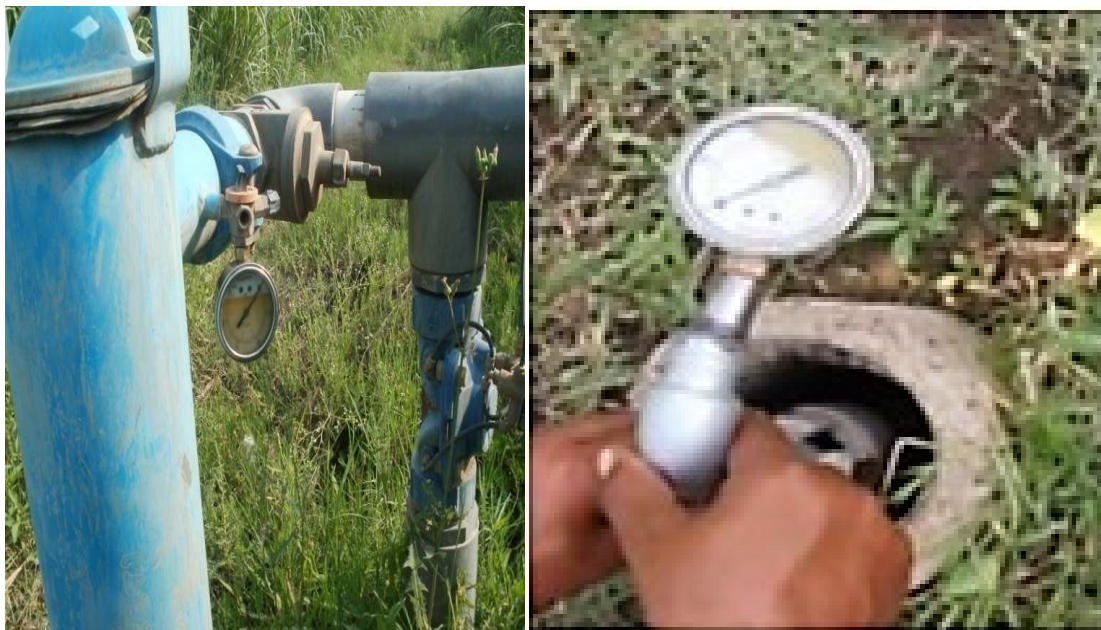
Appendix Picture 3. Pressure adjustment, measurement at the hydrant and riser valve using pressure gauge.
