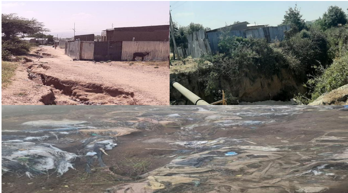
Figure 4.13. Sample photo of poor drainage in informal settlement and no drainage system
