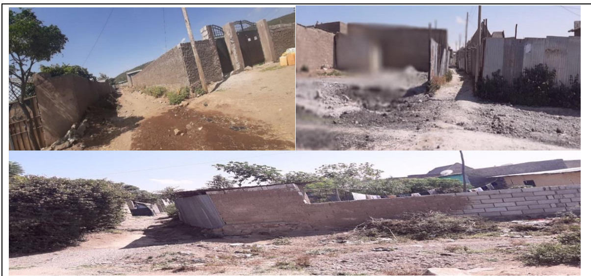
Figure 4.12. Road Condition In Informal Settlements (in Dagaga kebele (05))
