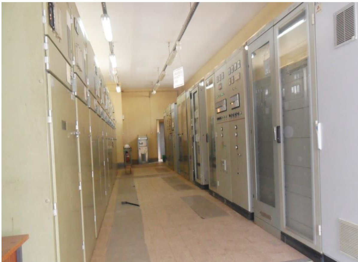
Figure 3. 3 Asella substation control room (source: researcher photograph)
