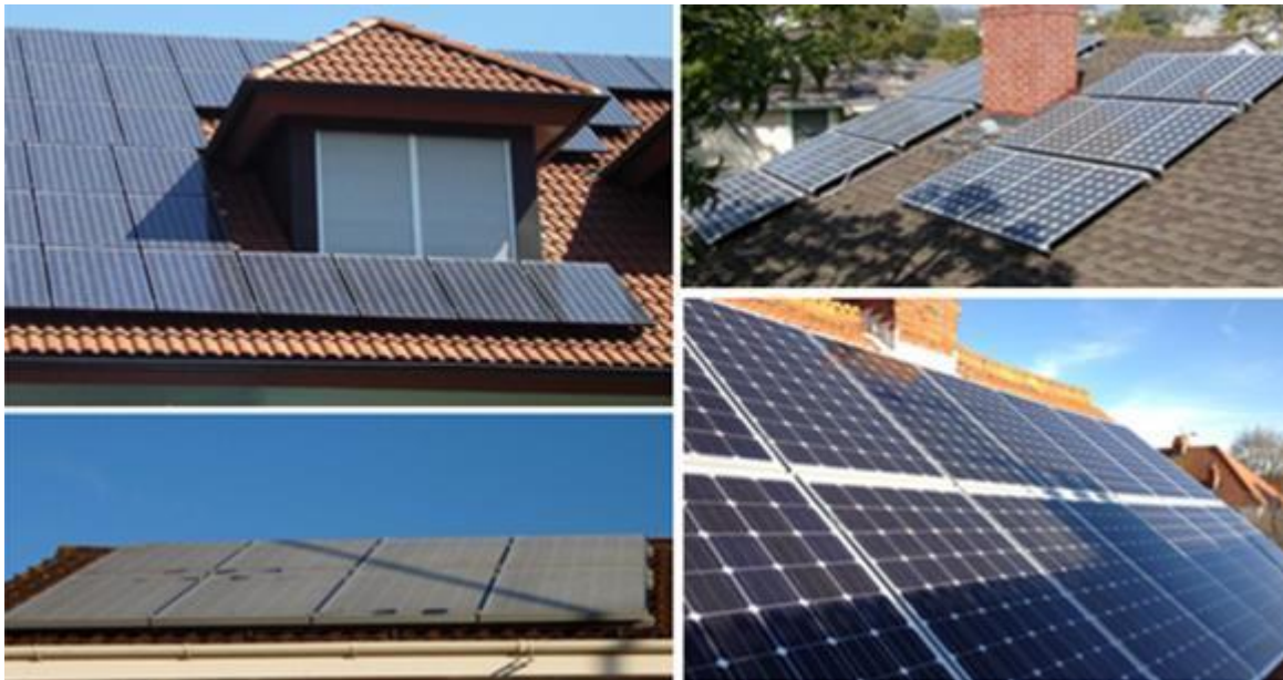
Figure 2.7 Partial shading on the rooftop PV module (Tzikas et al., 2017)
