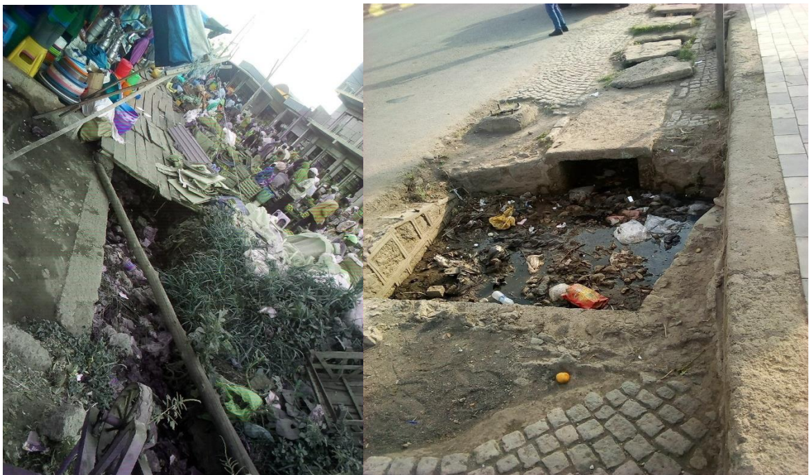
Figure 4.6 Lack of frequent clearance in the drainage system
