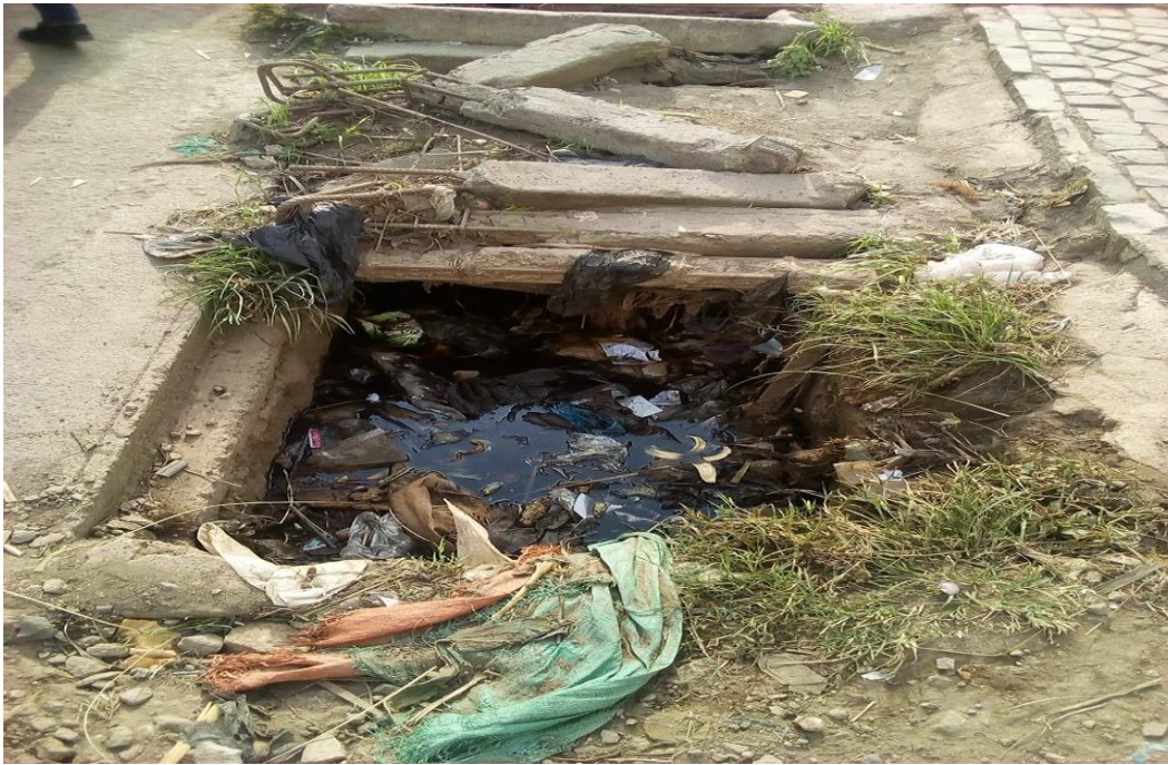
Figure 4.7 Damaged drain line
