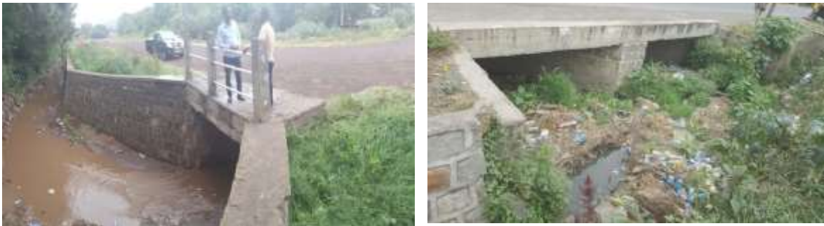
Based on the above figure there is almost 9 inlets which are properly constructed as well as not constructed. And also there is no waste treatment on the inlet as a chamber so these creates not only overflow of storm water it also brought overflow of liquid and solid wastes. Therefore, these affect the two ecosystem services of wetland that are source of freshwater and capture fisheries dependent on the natural reproduction.
