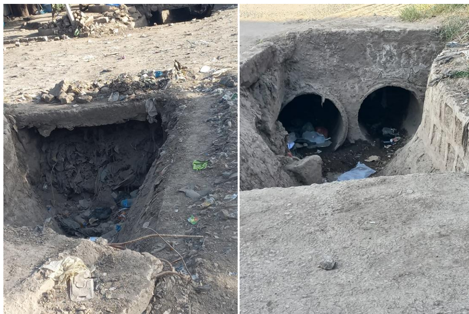
FIGURE 23: SITE C CURRENT FAILED CULVERTS
