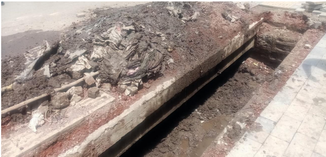
FIGURE 20: DRAINAGE BLOCKED BY MUD AT SITE B
