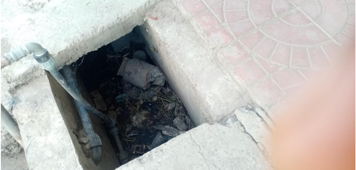
FIGURE 21: ILLUSTRATION OF DAMAGED MANHOLE COVER
