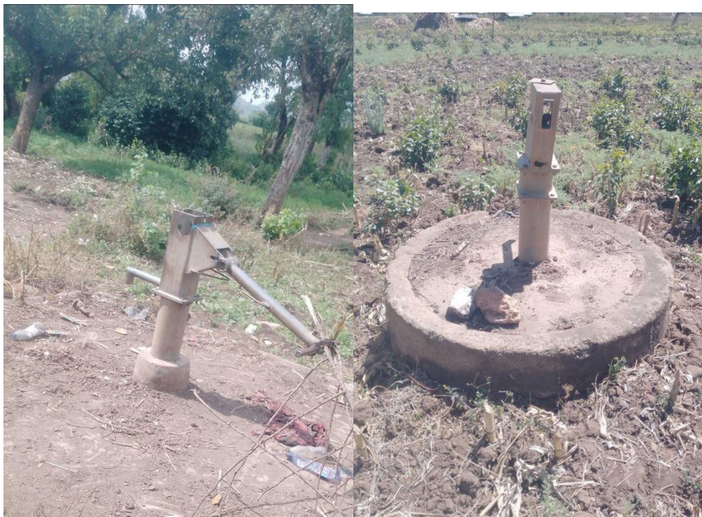
Figure 4.8 Lack of spare part and Tools non-functional schemes
