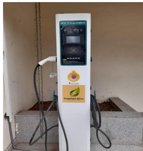
Figure 2.1: AC EV charger (Level 2)
