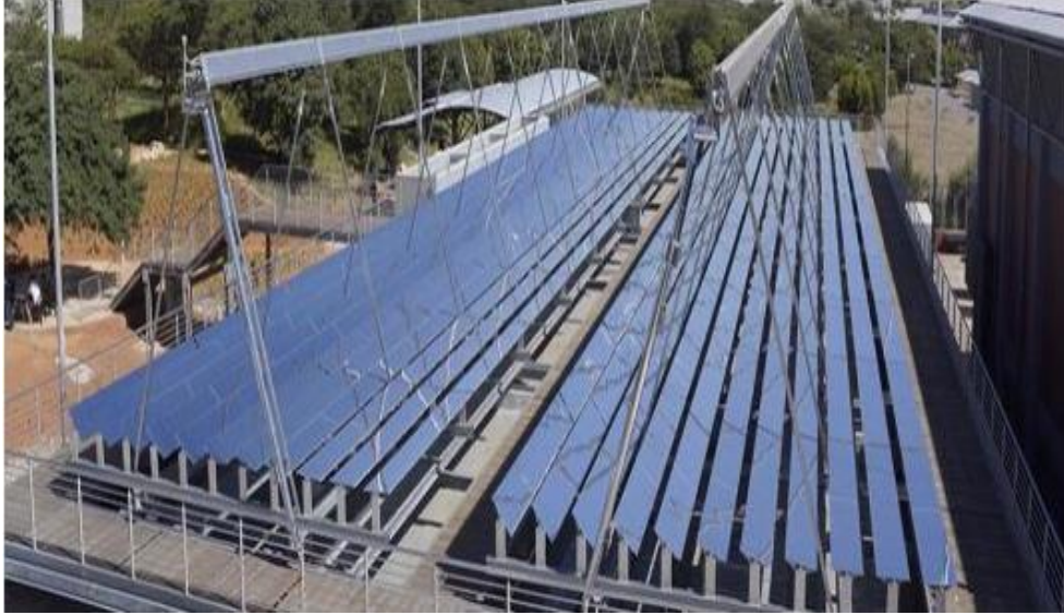
Figure 2.7: The roof-top installation in South Africa (Industrial solar)
