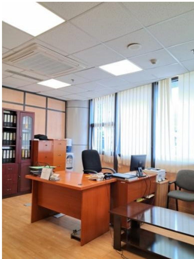
Figure 28 - The figure shows that 50×50 cm ceiling panel lights are used during the day in the office of the Nib Bank building (Source: Author march 12, 2025 at 9:00 AM LT)
