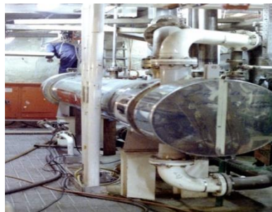
Figure 1. 1 Physical appearance of industrial shell and tube heat exchanger plant
