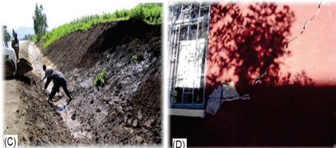
Figure 2. 7 (C) Roadside ditch clogging. (D) Cracks in the wall of a residential building (Arega, 2012).
