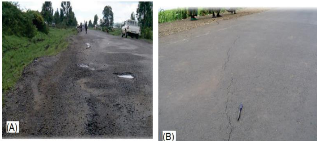
Figure 2. 6 (A) Road surface deformation and formation of potholes, corrugation, and ruts. (B) Formation of longitudinal cracks due to the presence of expansive soils.
