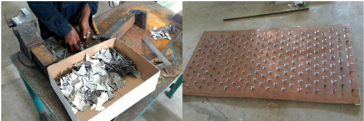
c) Manufacturing of the obstacles and planting it on the absorber plate
