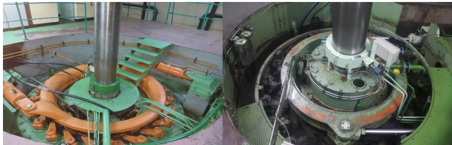
Figure 3.11 Turbine and servo system of Koka and Awash II HEPP
