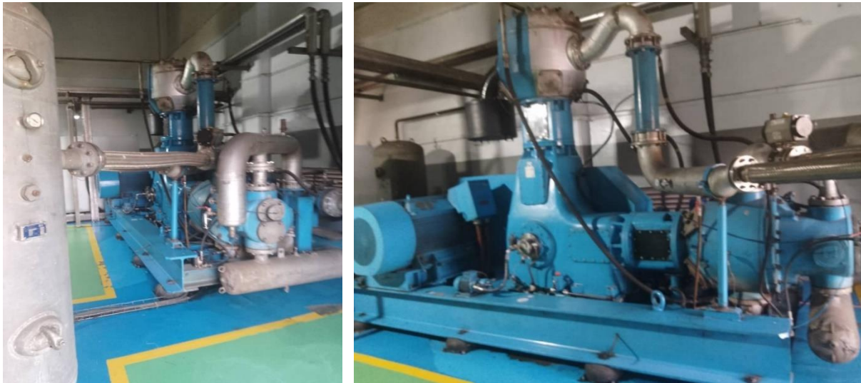
Figure 3.14 High pressure compressor
