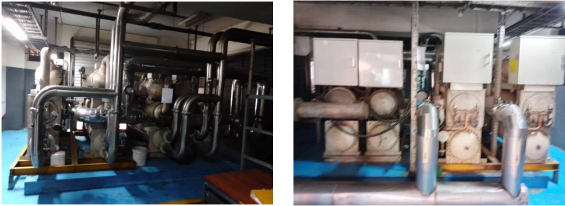
Figure 3.16 Water cooled chillers
