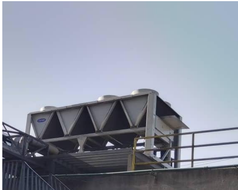
Figure 3.15 Air cooled chiller
