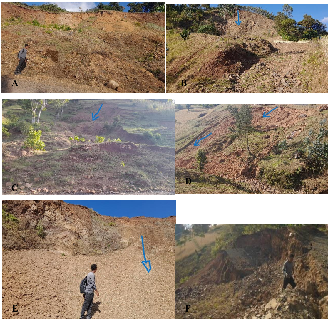
Figure 4. 3. Different field photo of study area affected by landslide (A) Complex, (B) Rock slide, (C) Debris slide (D) Earth slide, (E) Debris slide and (F) Rock slide type of landslides.
