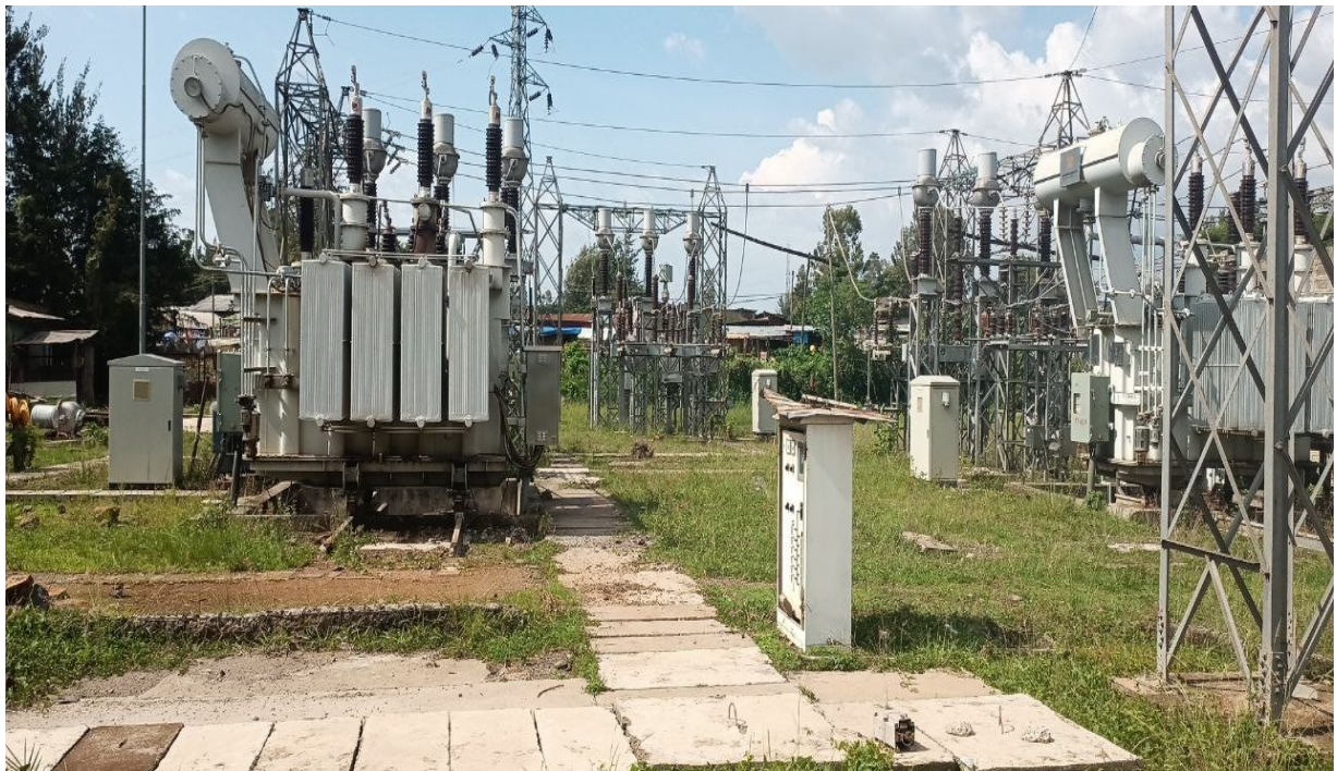
Figure 3. 2: Weliso distribution substation
