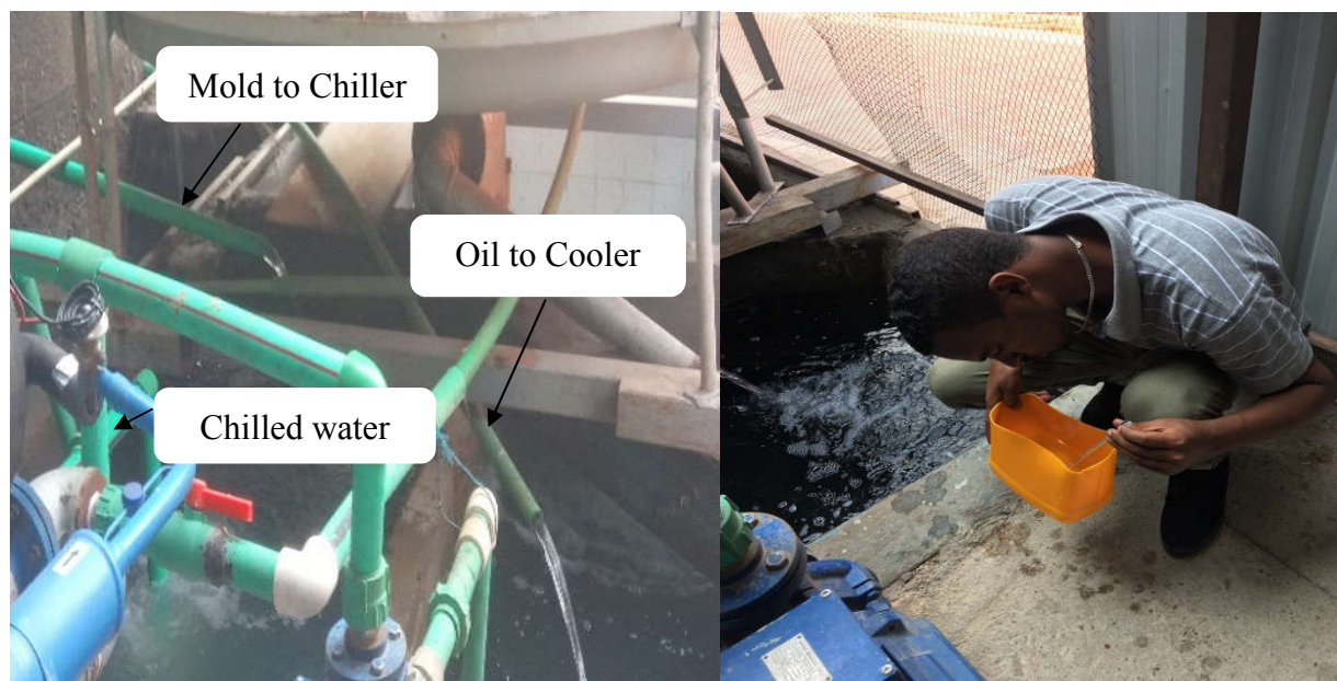
Figure 6. 2: Chiller temperature measurement in Bekas Chemical PLC
