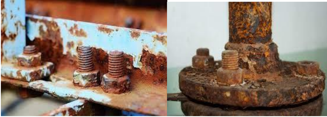
Figure 1.2. The corrosion effect on fasteners W.M. Tang et al. (2003)
