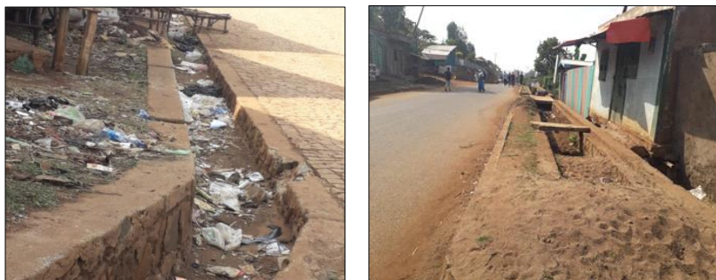
FIGURE 4.4: DETERIORATED AND BELOW STANDARD CONSTRUCTED DRAINAGE (Source: Field survey, 2021)
