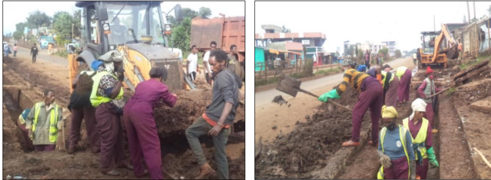
FIGURE 4.15: TEMPORARY SOLUTION BEFORE TAKEN CLEANING DRAINAGE CHANNELS (Source: Dambi Dollo town municipality, 2020)
