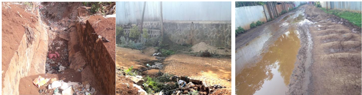
FIGURE 4.6: AFFECTED DRAINAGE SYSTEM AND STREET BY STORMWATER EFFECTS
