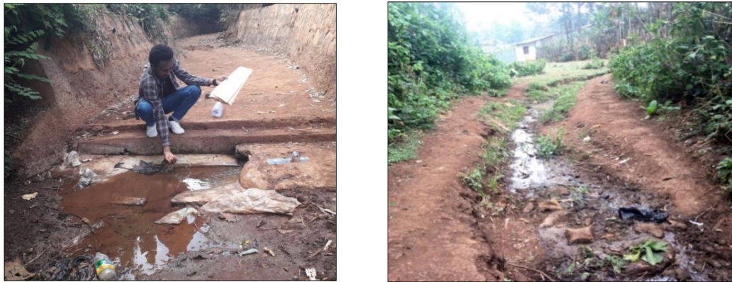
FIGURE 4.9: THE DRAINAGE CONNECTED TO THE RIVER AND BLOCKED BY SOLID WASTE
