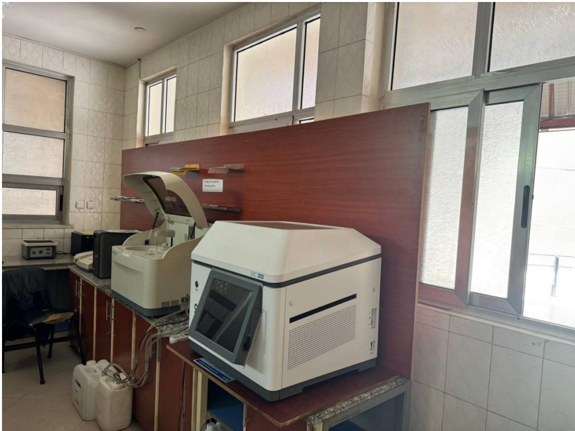
Figure 18 Laboratory with analytical equipment placed directly in front of a ventilation window.
