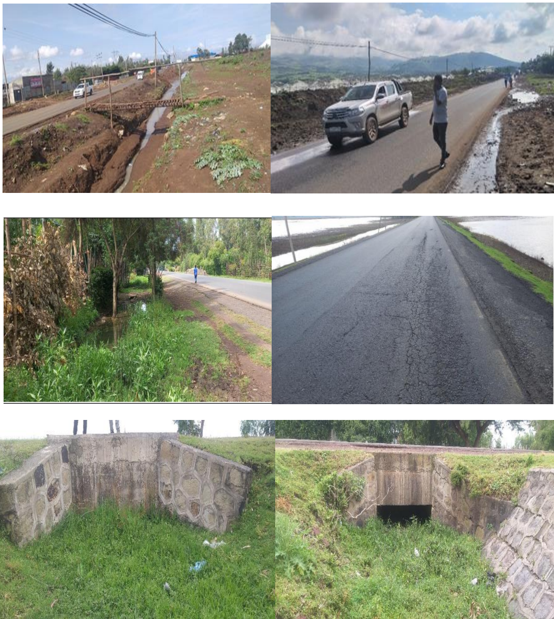
Figure 21: drainage problem along the road stretch
