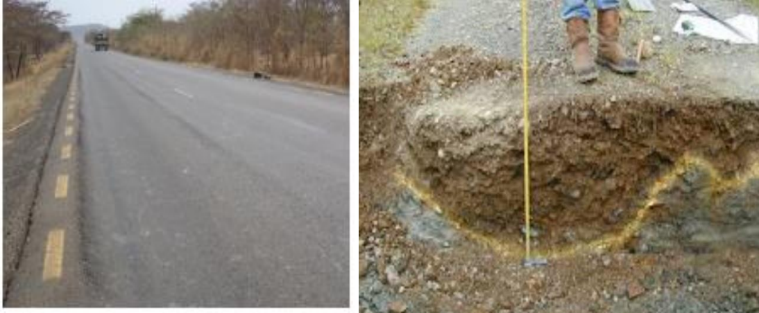
Figure 7: Rutting (Source: Google)
