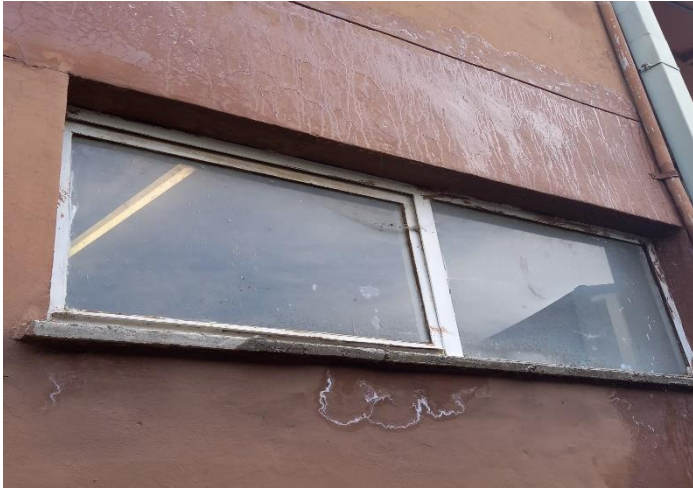
Fig 7. Leakage of water
