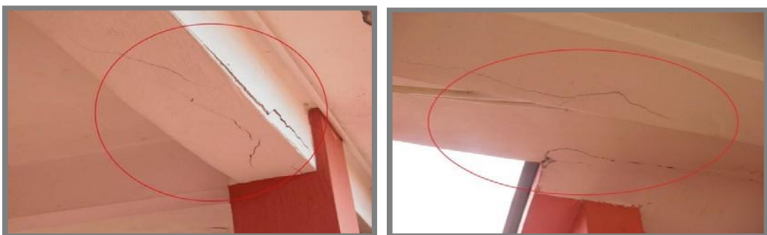
Fig 2. 1 Horizontal cracks (Othuman Mydin et al., 2014)
