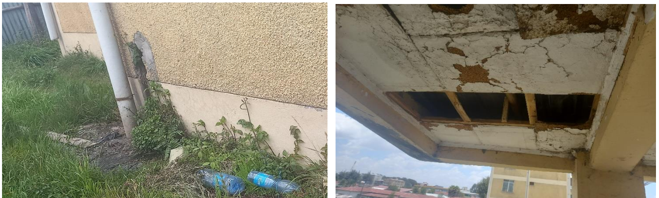
Fig 4. 18 Sewerage and Roof ceiling defects on building
