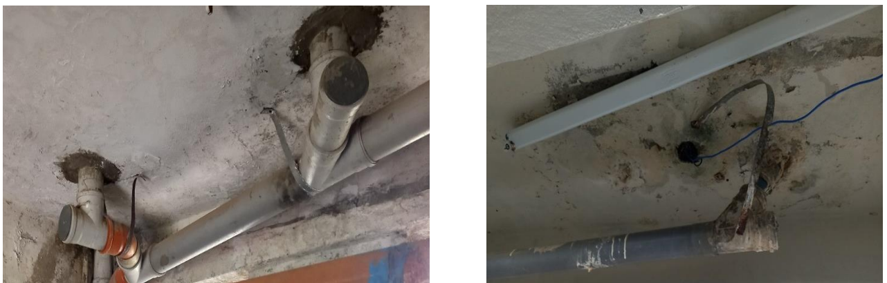
Fig 4. Plumbing and drainage defects
