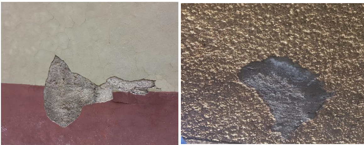
Fig 2. Defective plaster rendering on buildings
