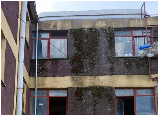
Fig 5. Fungi caused bay excessive dampness
