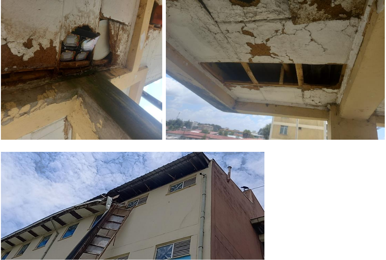
Fig 1. Roof and ceiling defects
