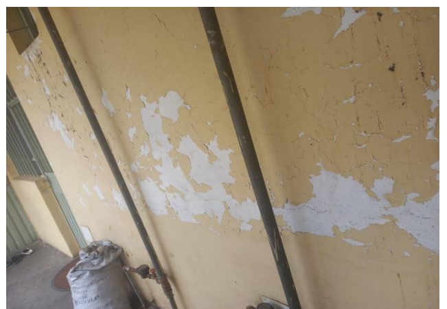
Fig 6. Peeling paint on wall
