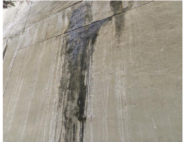
Fig 8. dampness on the wall
