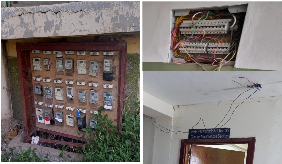
Fig 3. Electrical installation defects occur on buildings
