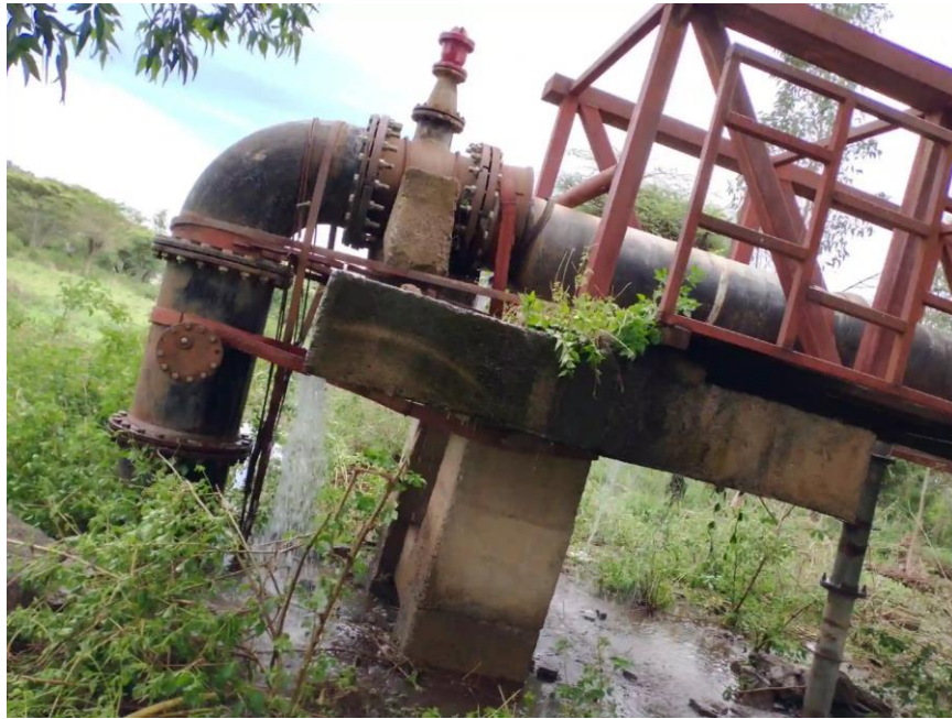
Image-1: Pipe Leakage on Transmission line at area called Shekla Factory
