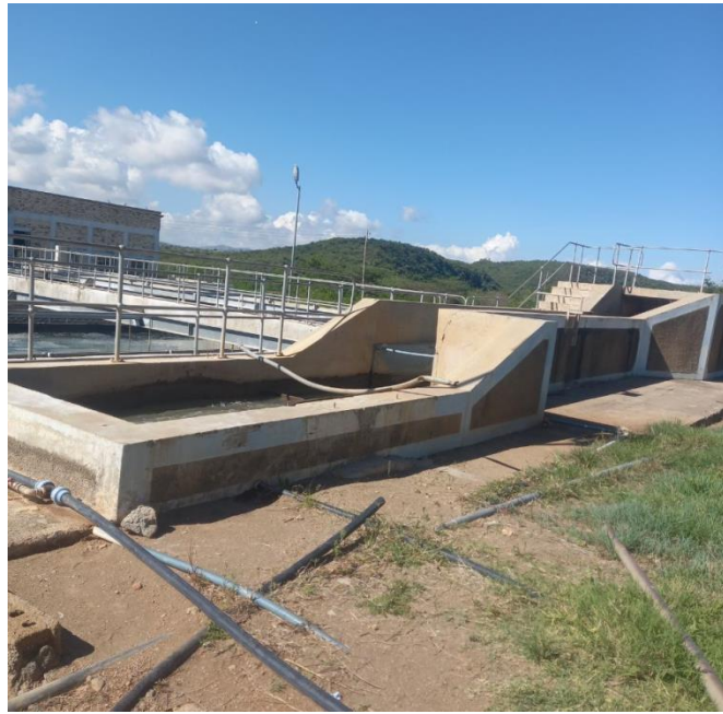
Image -3 Images of Water Treatment Plant at Koka
