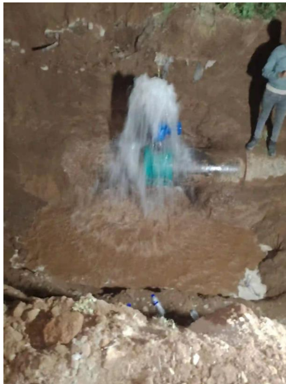
Image-2: Illegal connection in Kebele 09 caught due to pipe burst
