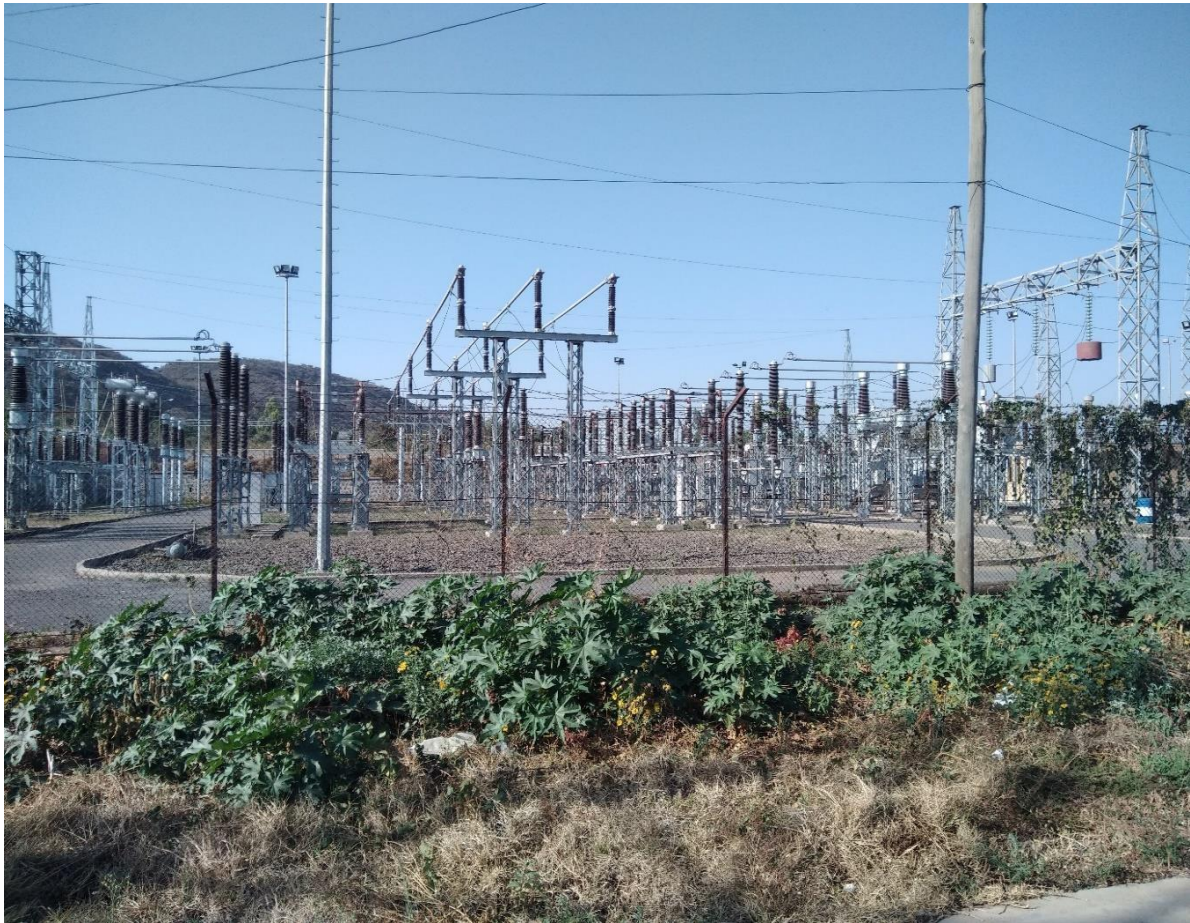
Figure 2. 21 Adama Distribution Substation
