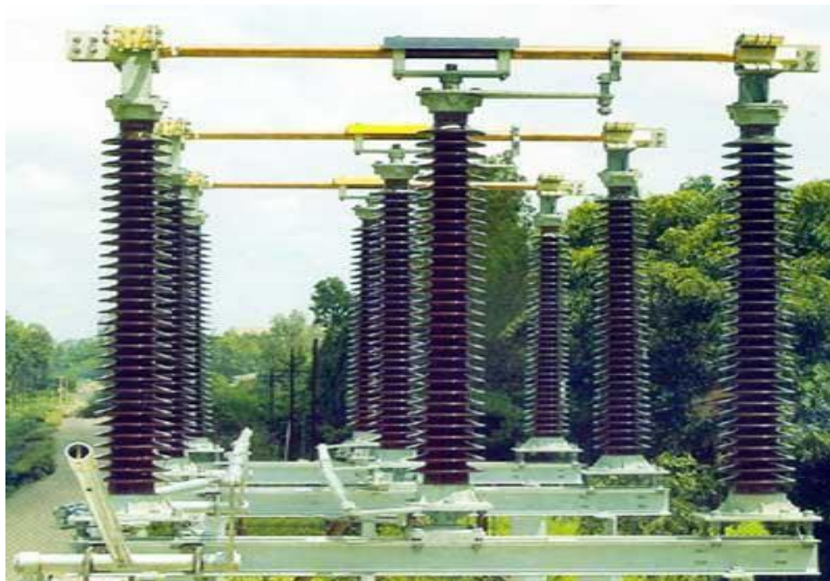
Figure 2. 23 Isolators in a substation
