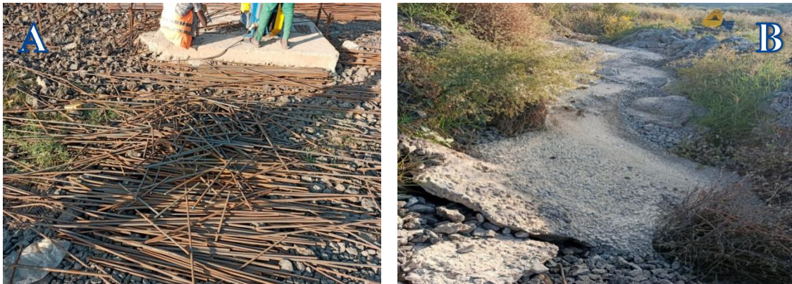
Figure 4.6 Wastes on Structural Works
