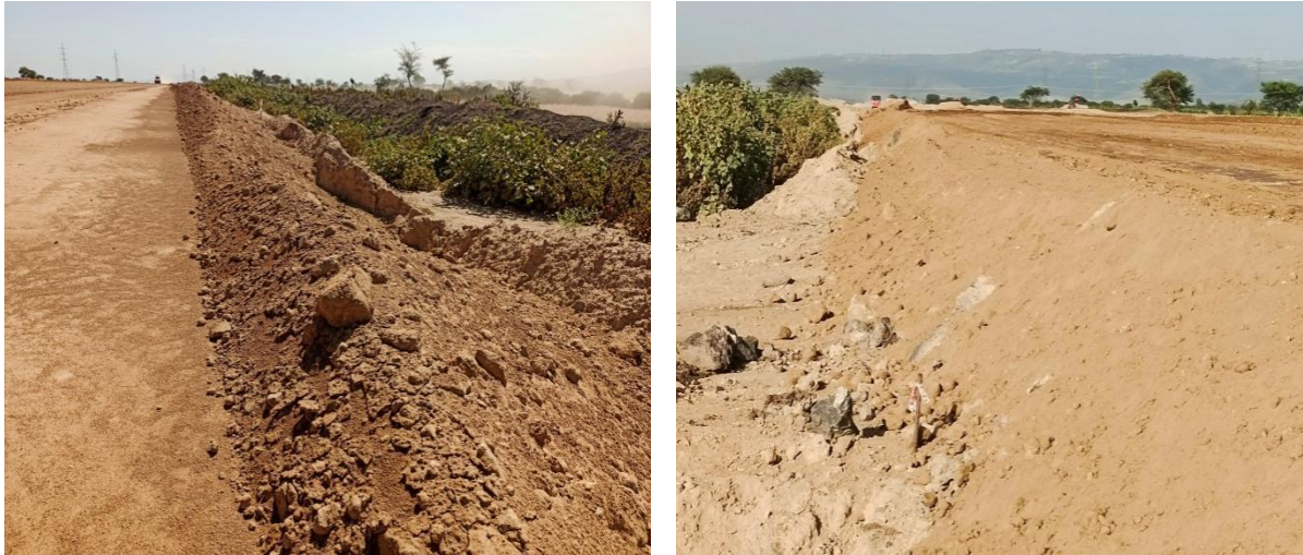
Fig1 Excess Capping Material
