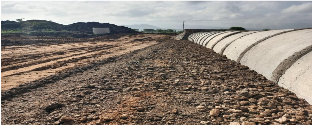
Fig 3 Using sub base material which is excess (using 1m width but 0.4m needed)
