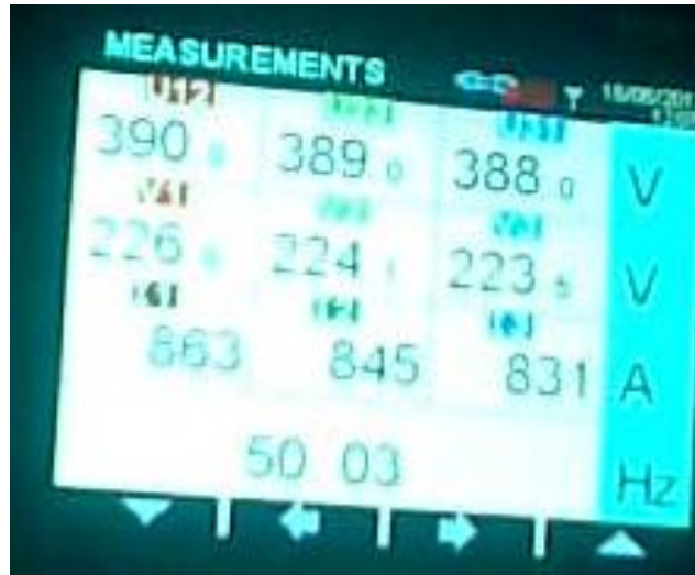
Figure A3 : Transformer7 1.6mva Transformer Load Profile Displayed on Power Stability Recorder
