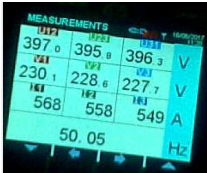
Figure A1. Transformer2 1mva transformer load profile displayed on power stability recorder
