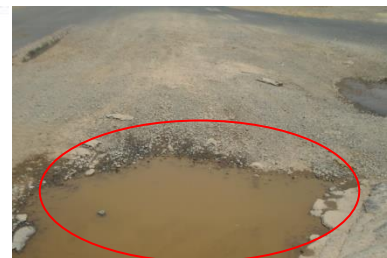
Potholes happened as a result of poor drainage system
