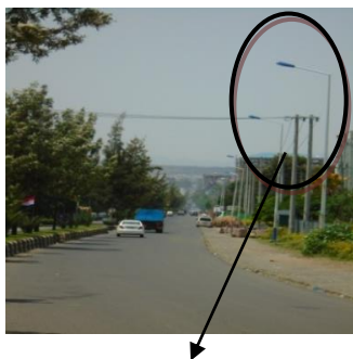
Un-functional street light
