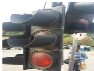
Un-functional traffic light
