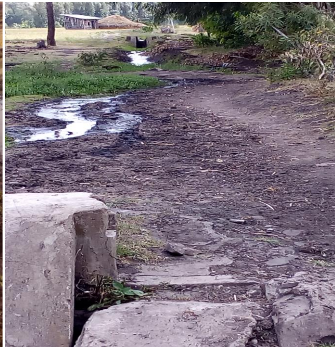
damaged drop structure
