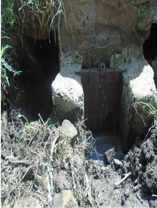
Damaged off take gate
