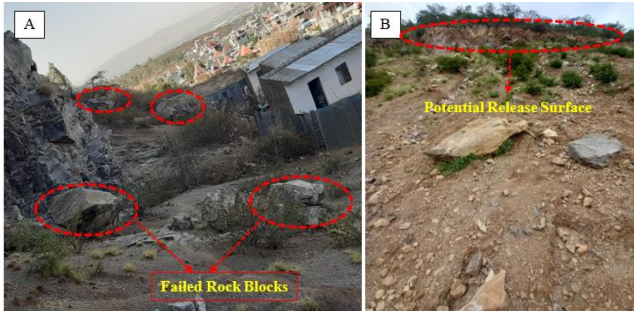
Figure 3. 1 Critical slope indicator A) Failed rock blocks and B) Release surface
